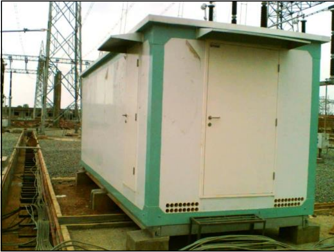
Power Sub station Kiosk
