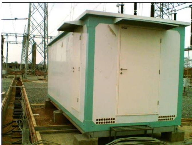
Power Sub station Kiosk
